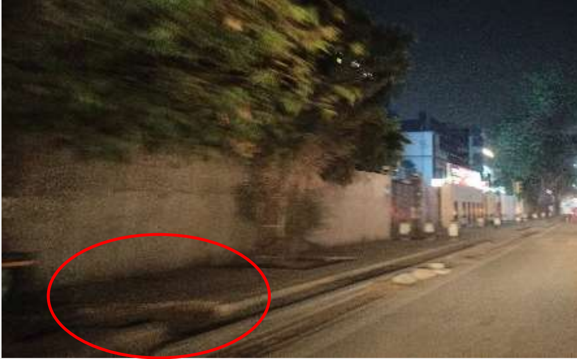
Vasant Kunj(2023): broken pavements
