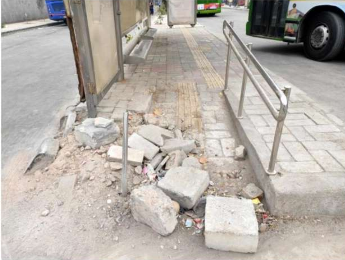
Broken ramp and tactile pavers at the waiting area
