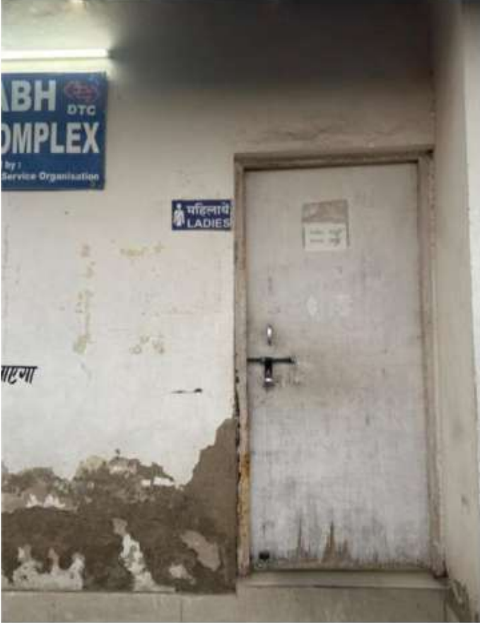
Limited access to women's toilet (keys available at the helpdesk upon request)
