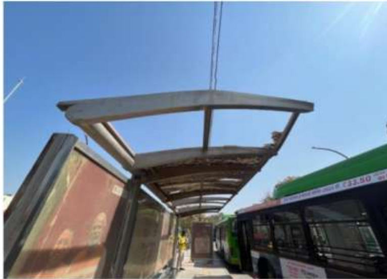
Broken shelter of the waiting area
