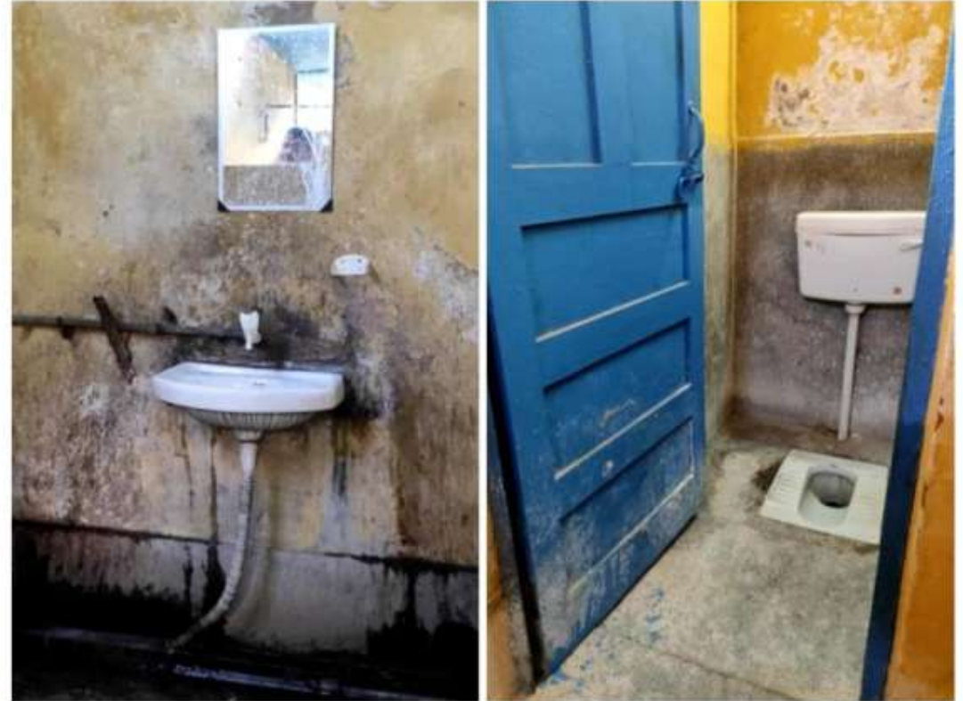
Washbasins and water closets are clean, however the facility lacks overall maintenance
