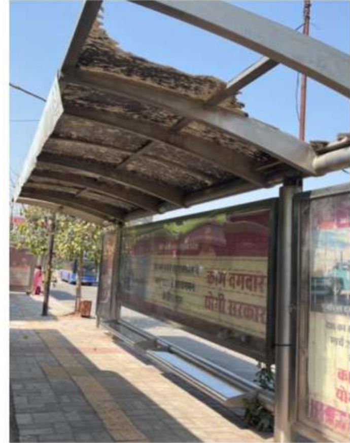
Broken shelter and lacks maintenance
