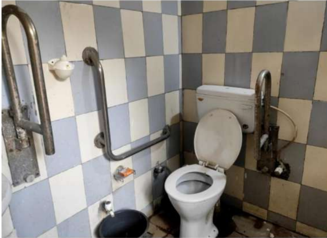
Provision of handlebars for PwDs, however lacks overall maintenance
