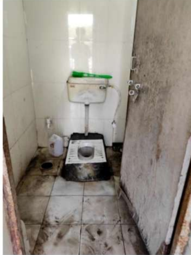
Unkempt water closet
