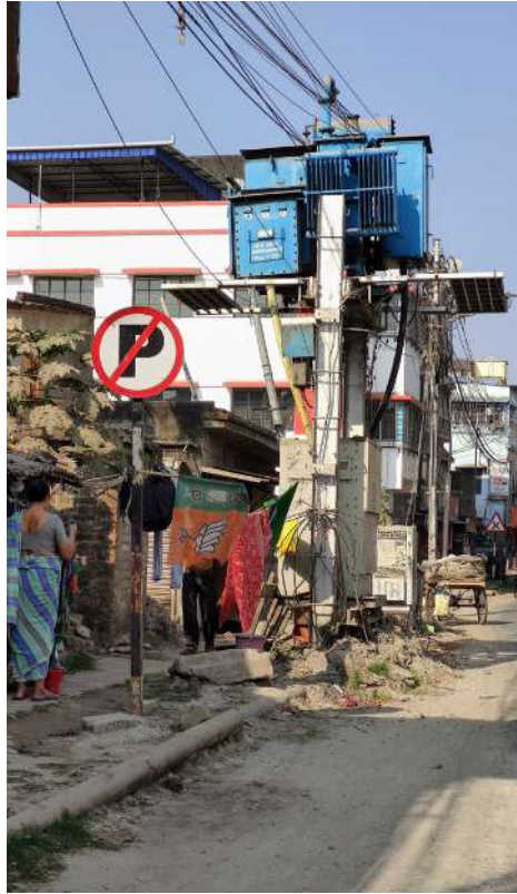
Image: Power transformers
